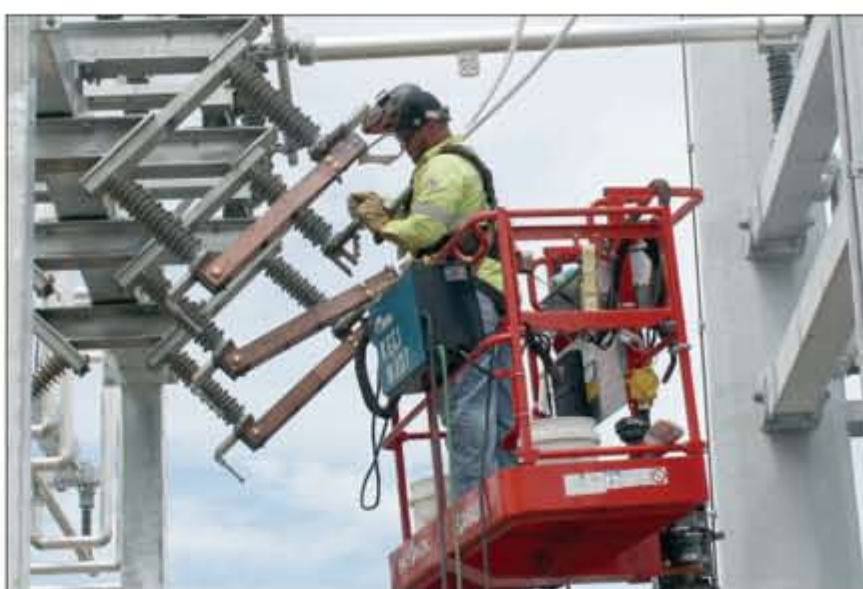
Michael Lunn with Koontz Electric out of Morrilton welds jumpers to the hook switches above the main breakers at the Cofer Road substation on Monday. The station is expected to be opened in late September.
