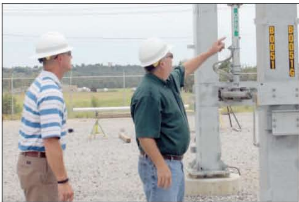
Entergy Arkansas Customer Service Representative Flave Carpenter (left) and Entergy of North East Region Engineering Supervisor Mike Willems look at equipment at the Cofer Road substation Monday. The addition of another substation will give Entergy three substations in Searcy.
